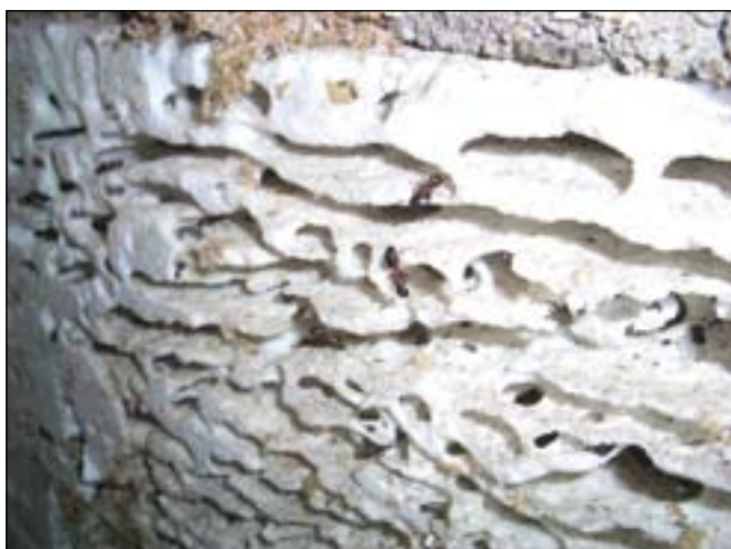
Damage in expanded polystyrene caused by Carpenter ants ( Camponotus ligniperda ).
